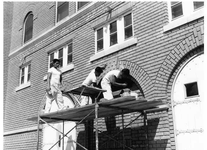
ABOVE: Students repairing a wall at Phoenix Indian School, n.d. Billie Jane Baguley Library and Archives, Heard Museum, RC284(1):1.320.
